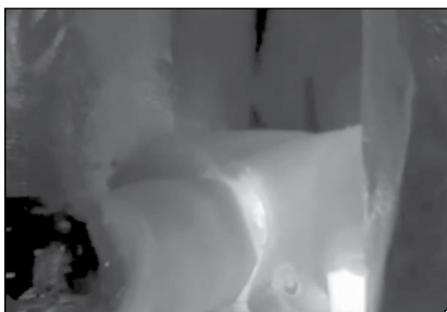
Leak in a 4-way valve dryer skid
